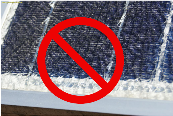
Broken glass, damage probably caused by impact, for example hail, stones, etc. 11
