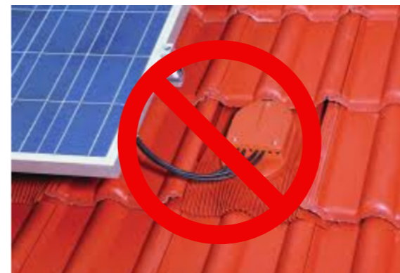
Example of improper cable installation 14
