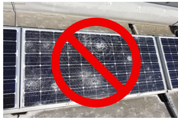
Damage after hail impact 12
