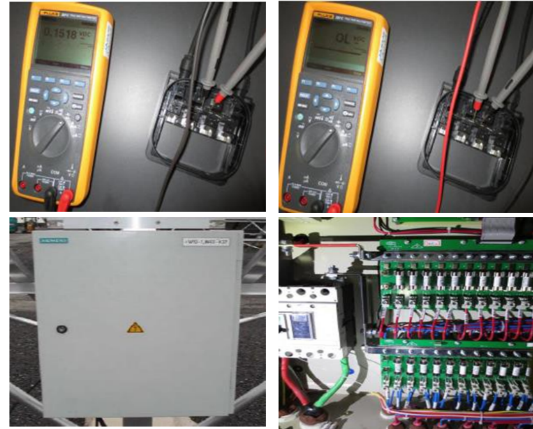
Electrical device for R iso , V oc , I-V curves:
